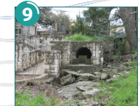
Stormwater outfall serving downtown Wimberley.
