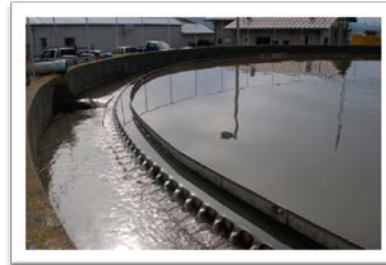
Figure 26. Wastewater treatment plant. Photo by Arcata Wastewater Treatment Plant & Wildlife Sanctuary, CA.
