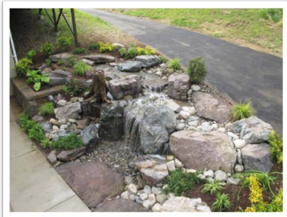
Figure 4. Pondless storm water waterfalls can be incorporated into stormwater drainage or rainwater catchment systems. Photo by BJL Aquascapes, LLC.
