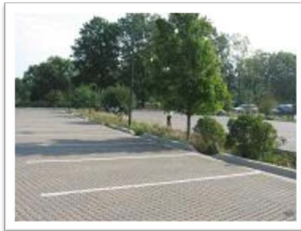
Figure 30. Pervious Parking Lot. Photo credit unknown.
