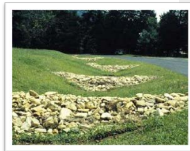
Figure 51. Rock berm installations on dry drainage area. Photo by Lake Superior Streams: Grassed Swales.
