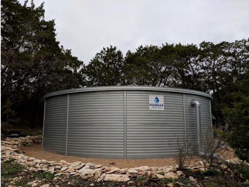
Figure 4. Rainwater Harvesting System installed at WVWA Headquarters
