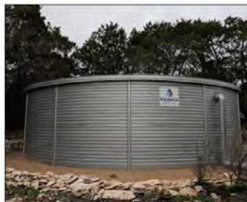
Rainwater Harvesting System installed at WVWA Headquarters
