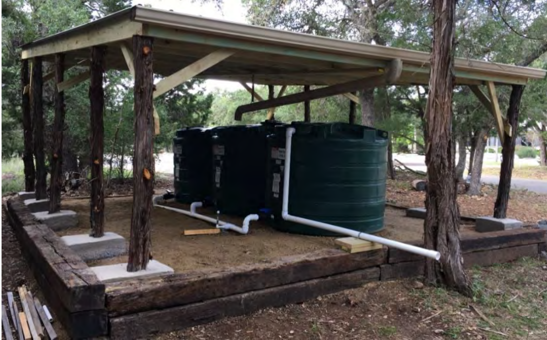
Figure 3. Rainwater Harvesting Systems installed at the Patsy Glenn Wildlife Refuge
